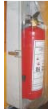
Fire extinguisher in box
