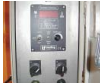
Computerized control of heating
