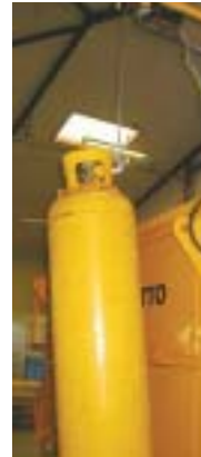
Crane for gas bottles
